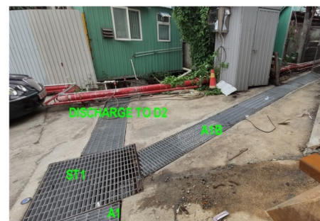
DRAIN A1, A1B, SANDTRAP ST1, AND DISCHARGE TO VILLAGE DRAIN D2
