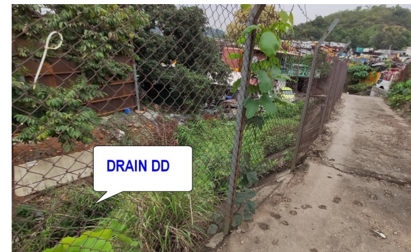
Photo 3 Condition of Drain DD, natural village stream
